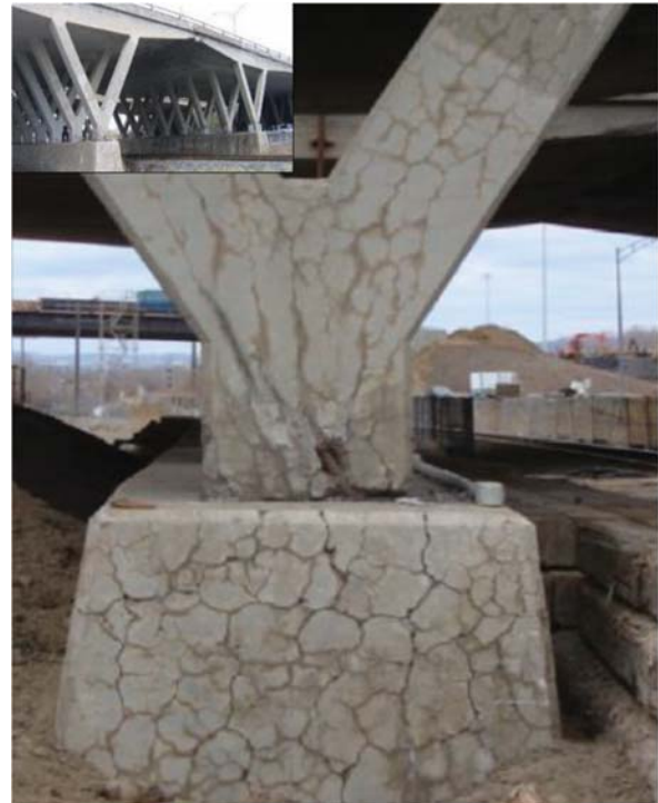
Fig. 1—ASR-affected column and foundation block of Robert-Bourassa/Charest Bridge, Canada, demolished in 2010 (taken from Sanchez et al. 6 ).
