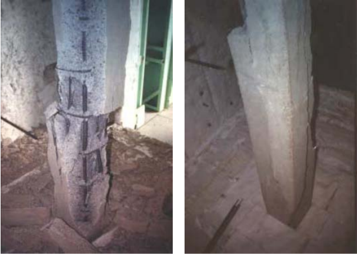
Figure 3-4 HSC-column (left) showing extensive spalling compared to a similar NSC-column (right) (Kodur and Sultan, 1998)
