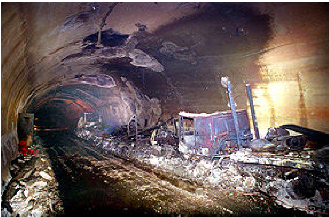
Figure 3-8 Damaged concrete in Mont Blanc Tunnel due to fire (Høj et al., 2008)
